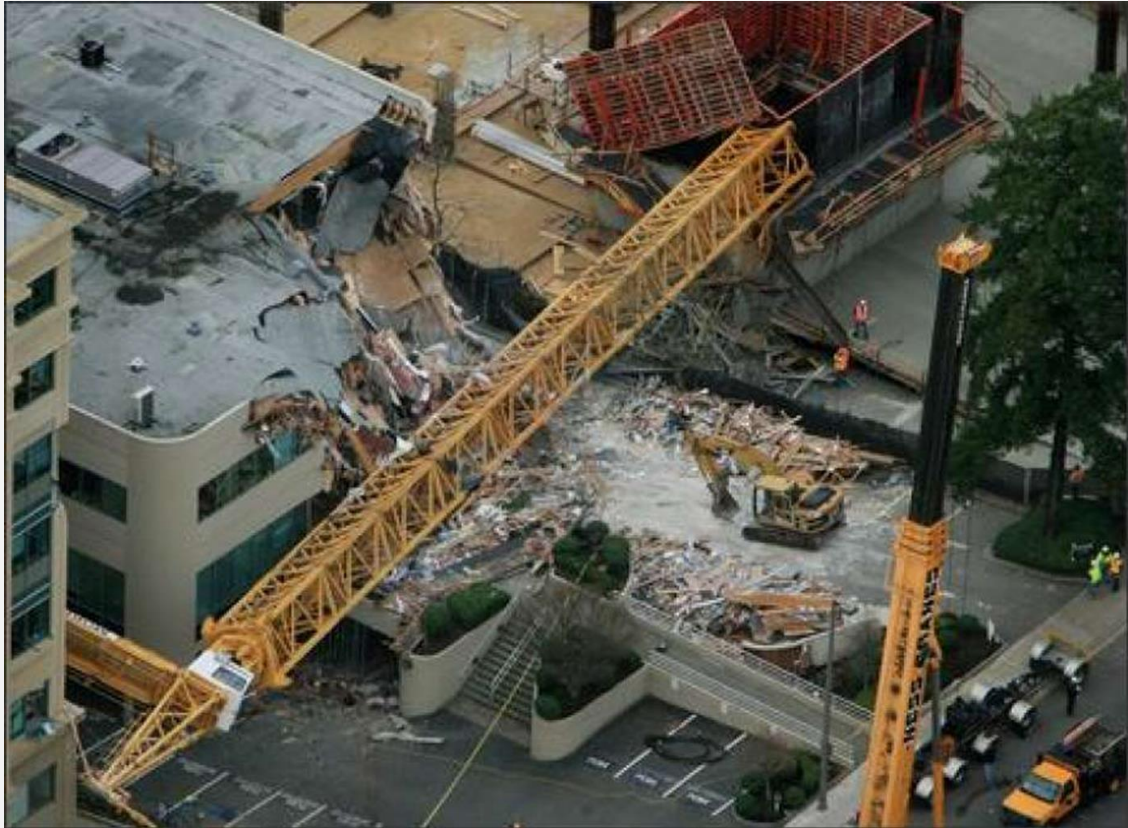
Tower Crane Collapse – Bellevue WA 2006. Structural engineer cited for errors in design. The citation was vacated in court.
